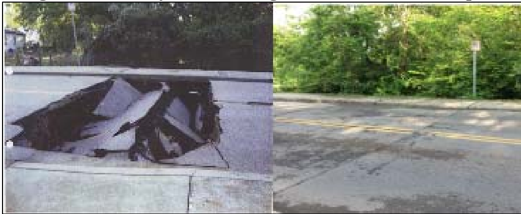
Figure 1: County Road Damages Before and After Repairs
