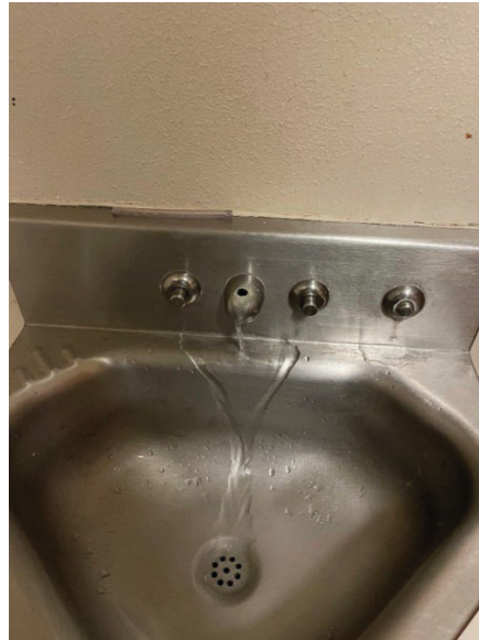
Figure 1. Broken Sink in Segregation Cell, Observed on July 31, 2024
