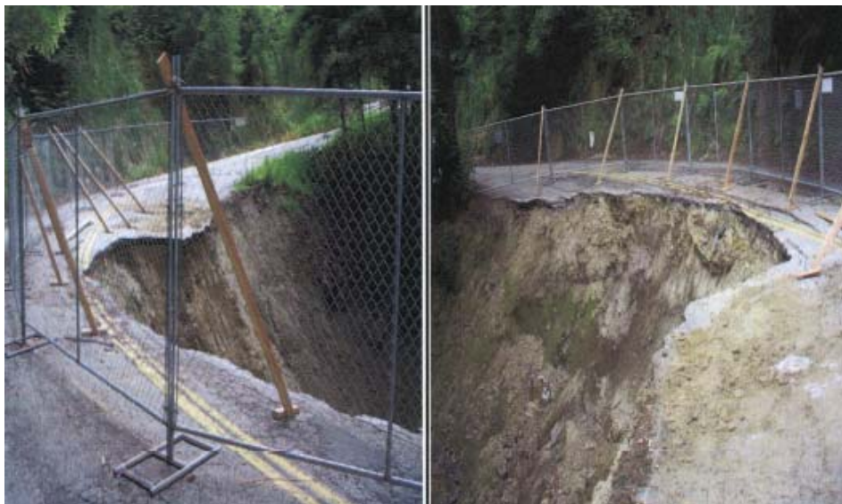
Figure 1: Project 268, Santa Cruz County – road damage at two sites of Vine Hill Road Source: Santa Cruz County
