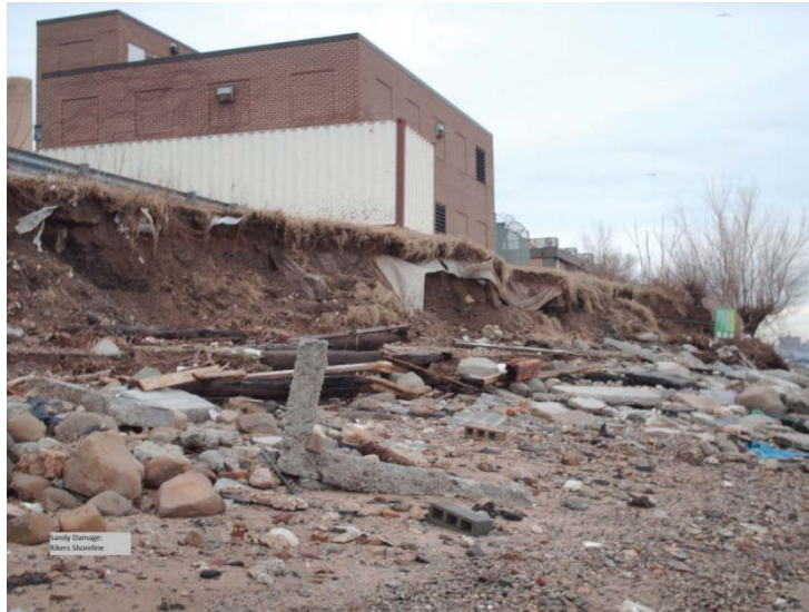
Figure 1: Damage to Facility at Rikers Island, New York
