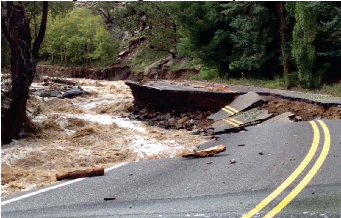
Figure 1: Damage to Fourmile Canyon Drive
