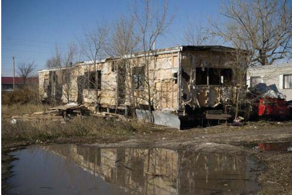
Figure 1: Damaged Home on Pine Ridge Indian Reservation
