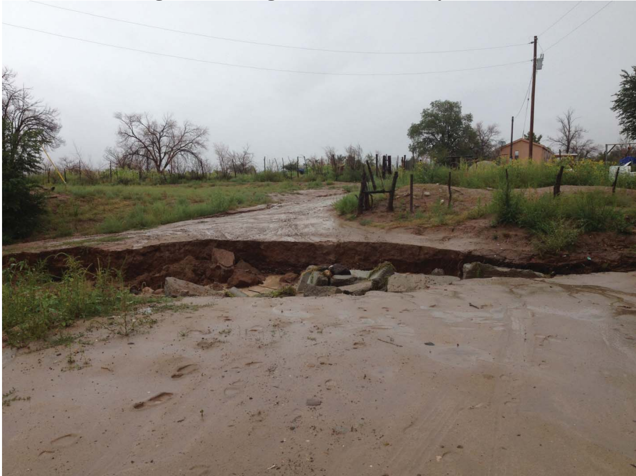
Figure 1: Damaged Road after Heavy Rains
